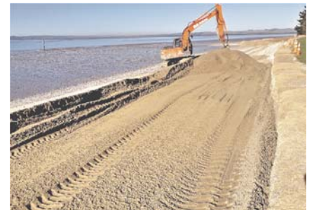
Shelly Beach, stabilised sediment backstop seawall and imported sand being placed (Photo: Christoph Soltau, Auckland Council).
