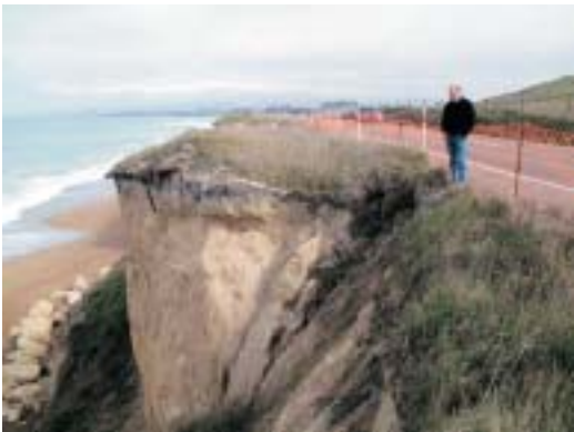
The Oamaru coast has eroded rapidly in recent years. The road at All-Day Bay has been moved twice over the last 30 years. The current proposal is to shift the road again, which may or may not be there in October, and place rock at the base of the scarp.
