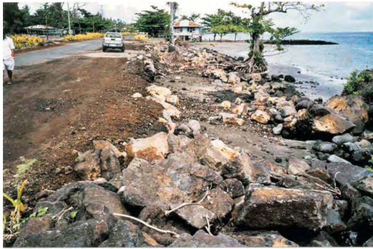
Figure 2: An example of a riprap seawall and road pavement failure in Savai'i. The land adjacent to the road has eroded some 8 to 10 metres inland.
