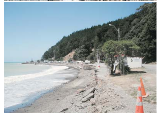
Rapid erosion of the shoreline in front of Clifton Motor Camp following removal of an old, failing and non-consented seawall in November 2009. Photos (top to bottom): Prior to November 2009; August 2012; prior to November 2009; January 2013 (note loss of row of trees and caravans visible in previous photo).
