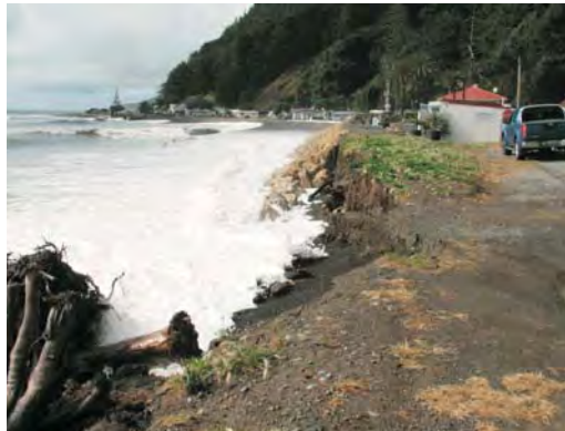
Erosion has continued on the downstream side of the Clifton Motor Camp's seawall. Photo: HBRC.
