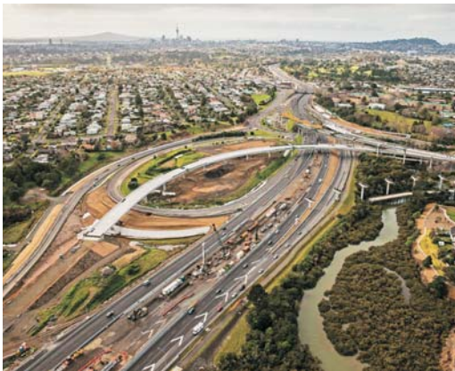
The Waterview Connection Project is the missing link that completes the Western Ring Route in Auckland. Photo: Well-Connected Alliance.
