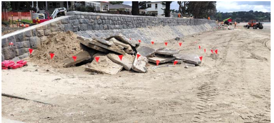
Ōrewa walkway and seawall project: Beach access ramp from Kohu Street and new shared path behind the seawall (top) and completed wall section extending north from the Marine View boat ramp (bottom).
